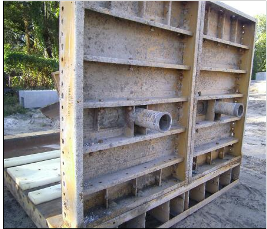
Steel Formwork for a Large Column Note the form liners which produce architectural features on the finished product
