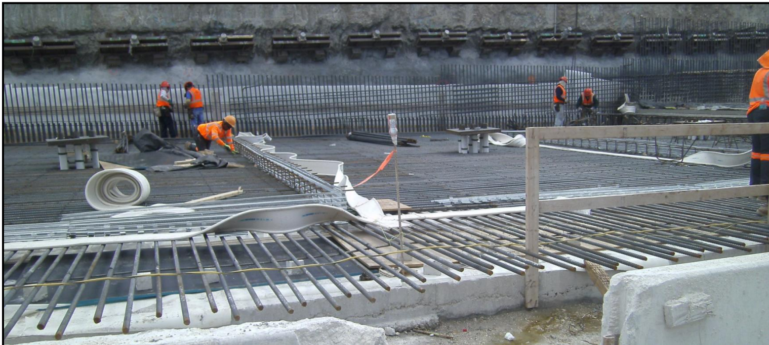
Where extensive mats of large diameter bars are used, reinforcing support is especially important. Note the use of mortar blocks to support the bottom mat.
