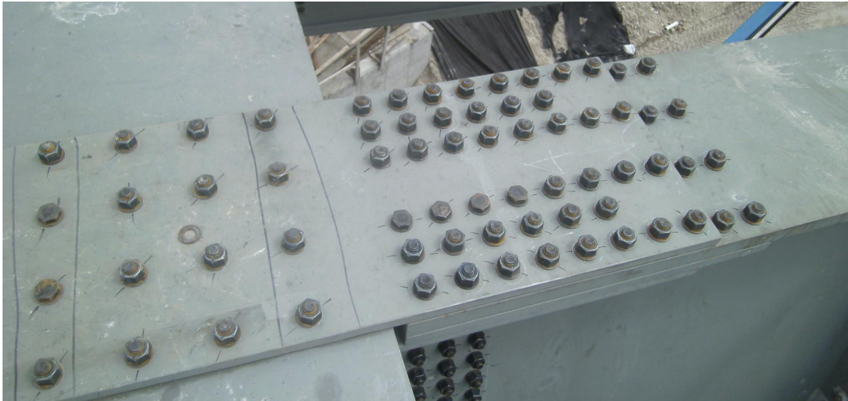
Splice Plate Connection – Note the markings where the “Turn of Nut” rotation was recorded
