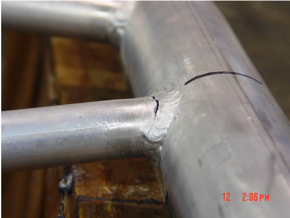
Figure 3: Fracture at base of weld – 4043 filler wire
