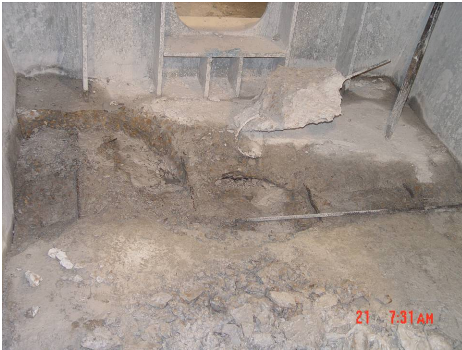
Figure 7: Concrete Failure (Removal of Loose Pieces)
