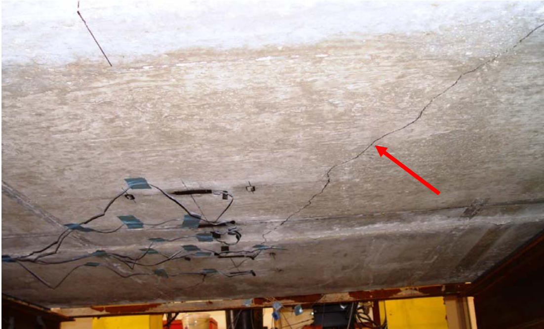
Figure 11 – Diagonal Crack after Continuous Load Test
