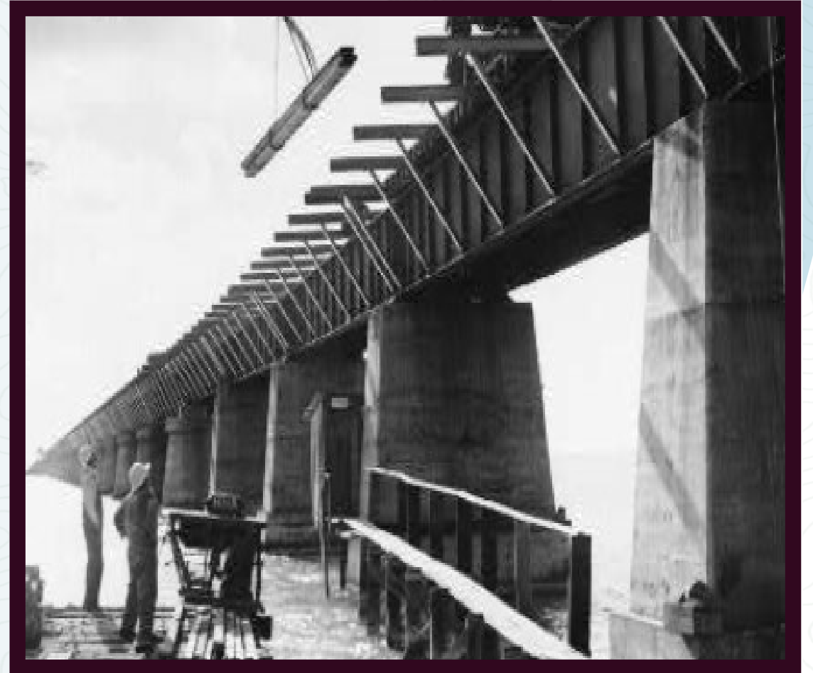
Cross Bracing of Floor Beams to support widening from Railroad to Roadway Bridge
