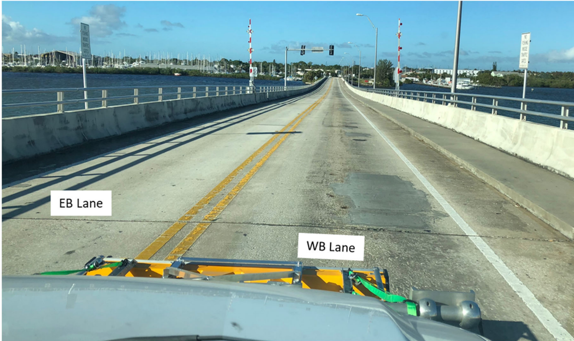
Figure 19: General view of St. Lucie bridge deck. Camera pointing West. Vehicle positioned ~50 ft. to the west from the bascule span.
