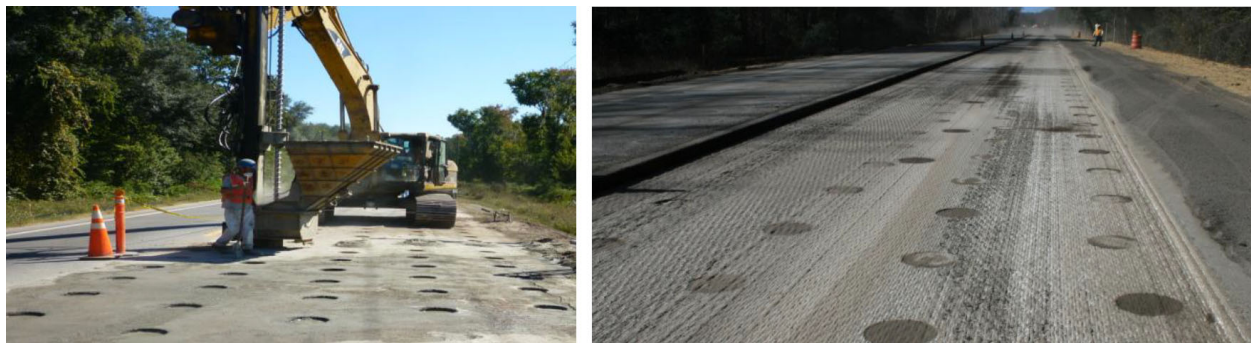
Figure 9: SSC installation grid layout on SR 100 (left); roadway surface after the milling (right) [5].
