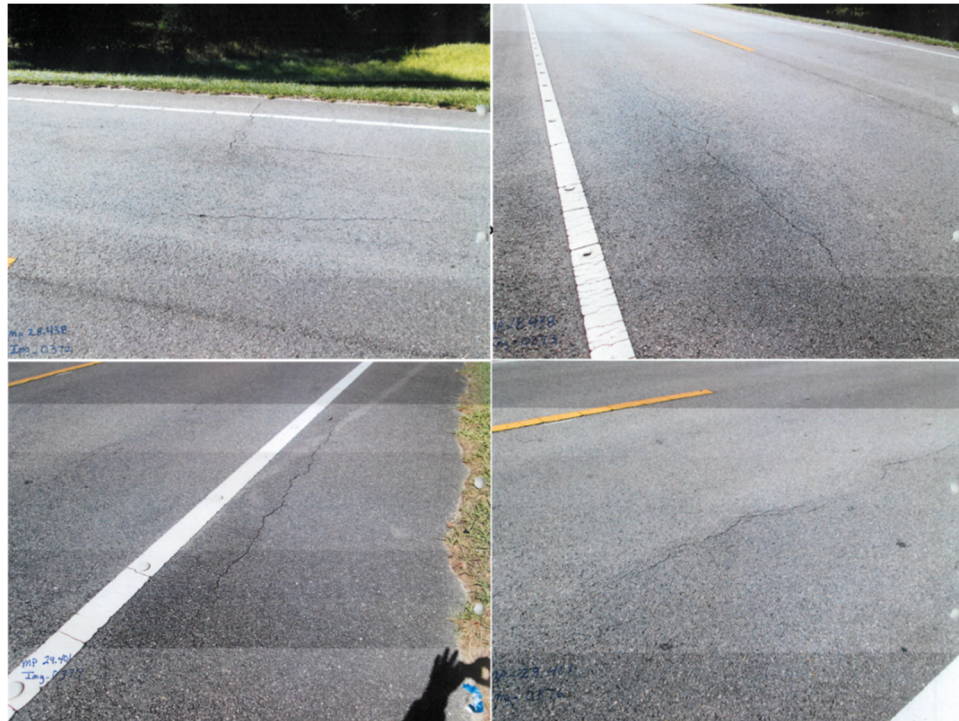
Figure 78: Photographs of pavement distress in proximity of MP 28.438 (top) and MP 29.401 (bottom).
