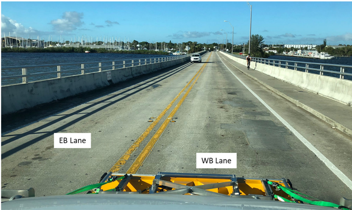
Figure 20: General view of St. Lucie bridge deck. Camera pointing West. Vehicle positioned ~450 ft. to the west from the bascule span.
