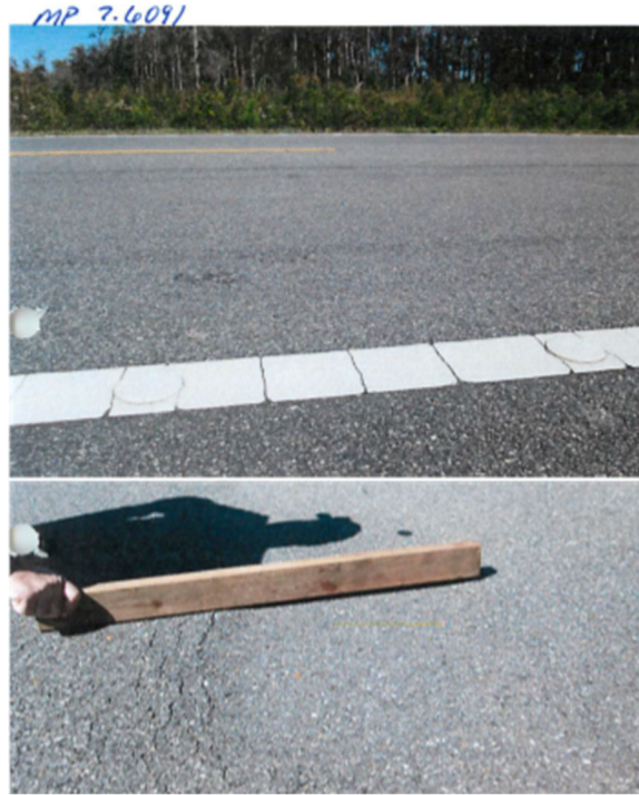
Figure 68: Photographs of pavement distress in proximity of core extraction point (MP 7.6091): a view of the lane (top) and signs of the distress on the pavement surface (bottom).
