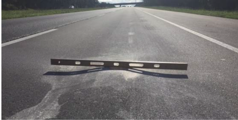
Figure 11: Observed rutting over the test section on I-10.
