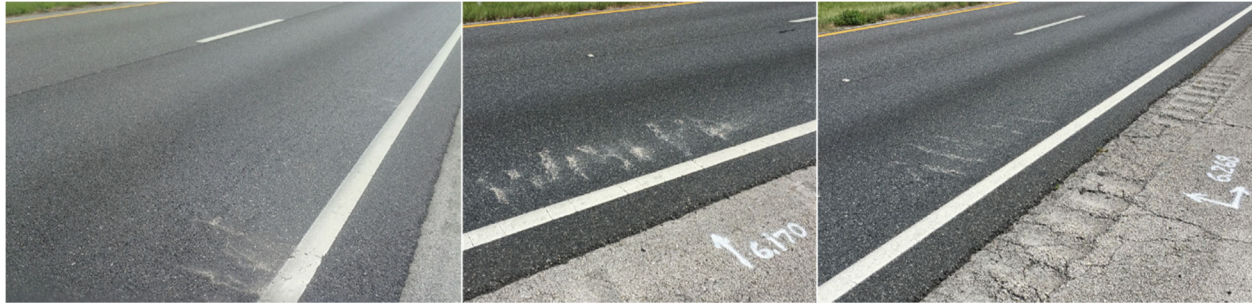
Figure 4: Photographs of eastbound pavement section R2 in proximity of core #1 extraction point at MP 0.123 (left); eastbound pavement section R2 in proximity of core #3 extraction point at MP 6.170 (center), eastbound pavement section R2 in proximity of core #4 extraction point at MP 6.268 (right).
