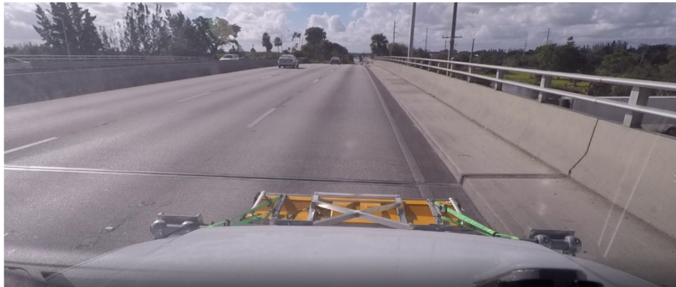
Figure 15: General view of Broward bridge deck. Westbound lane, right side. Camera pointing west.
