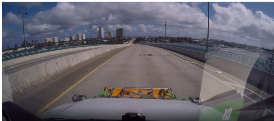
Figure 18: General view of Blue Heron Bridge. Eastbound lane, left side. Camera pointing East.
