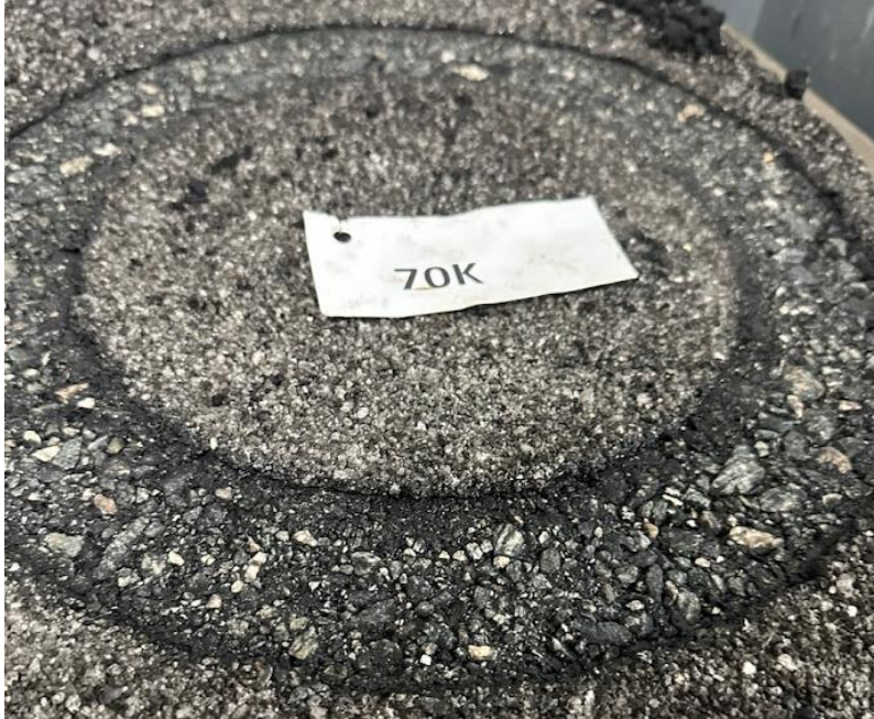
Figure 41: Loss of Aggregate in Wheelpath of Slag HFCS
