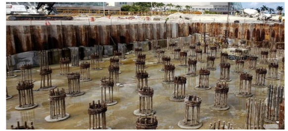
To be completed in 2027, the I-395 signature bridge will be 1,025ft long and span over NE Second Avenue and Biscayne Boulevard. The center pier construction will include 128 piles (3 ft in diameter with 27-in cages and extend approximately 120 ft below existing grade) as captured here in this image.
