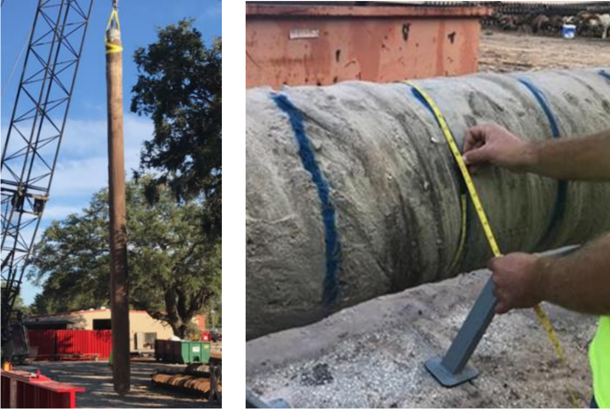
Figure 2.13 Pile completely extracted using crawler-crane (left) circumference measurements taken at 1-foot intervals along pile length (right) (Marinucci & NeSmith., 2017)
