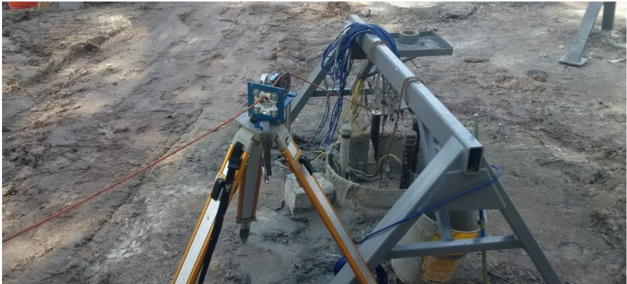
Figure 1.9 Infrared sensor probe being lowered into an auger cast pile access tube (Mullins & Johnson, 2017)
