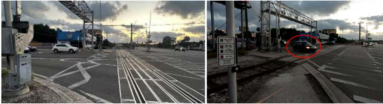
Figure 6-37. One-side RDE Pavement Marking at E Busch Blvd @ N Nebraska Ave. District 7
