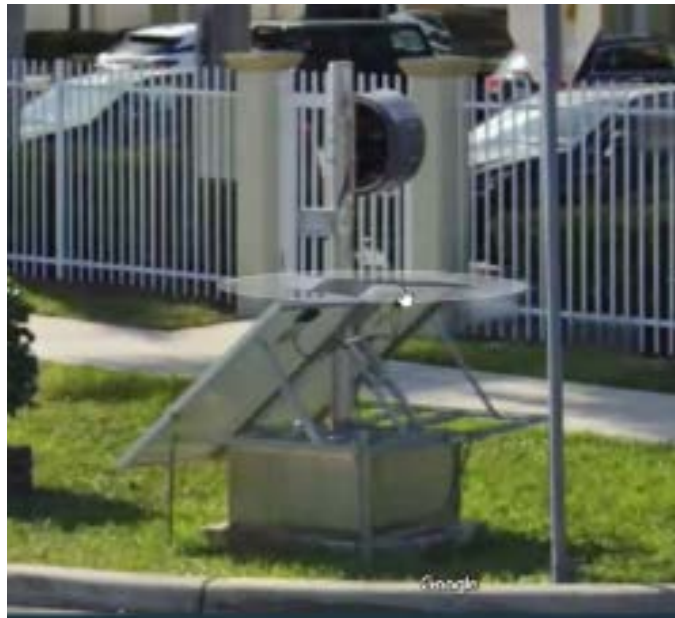
Figure 5-9. Brightline Violation Warning System in Miami, Florida
