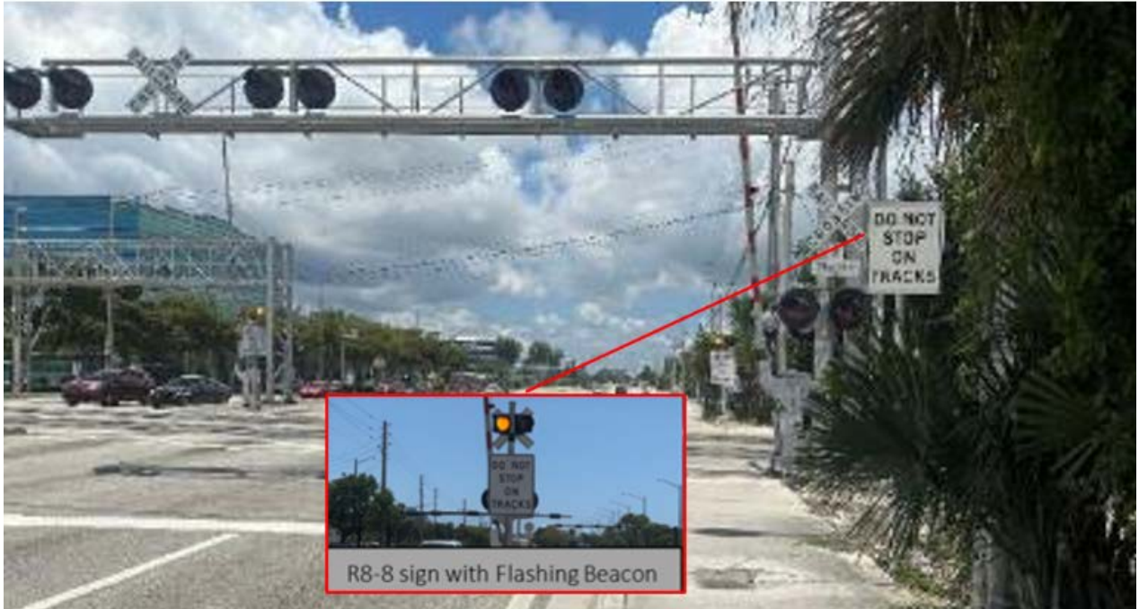
Figure 6-24. Suggested Countermeasure of R8-8 Signs at W Cypress Creek Rd @ N Andrews Ave, District 4
