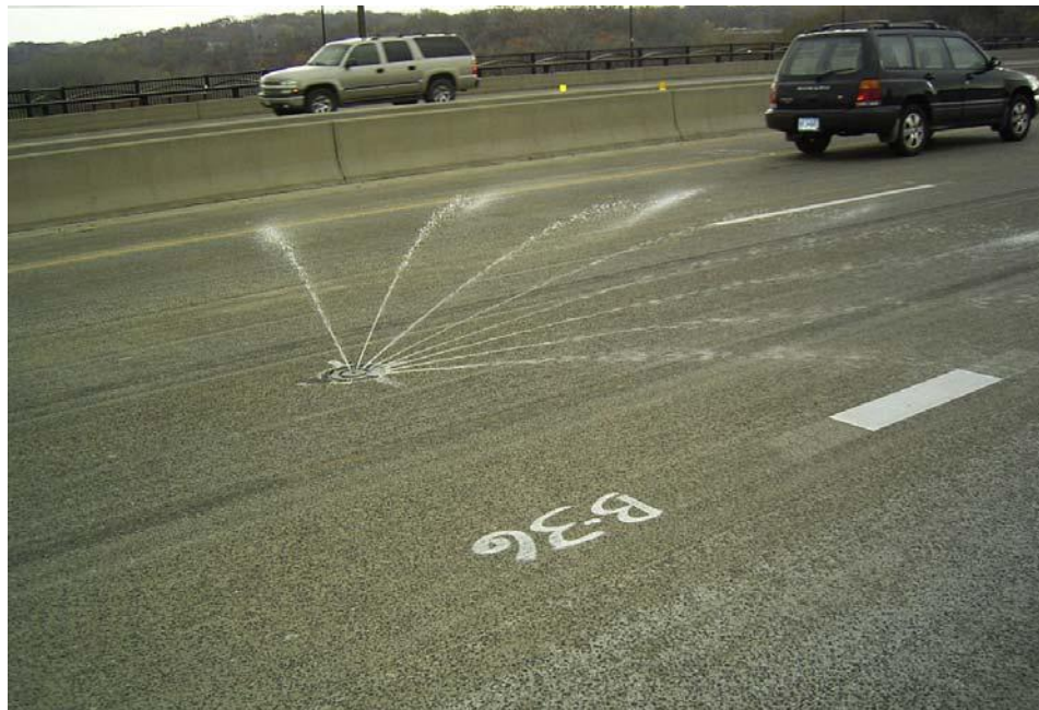
FIGURE 45 Anti-icing system on a bridge.
